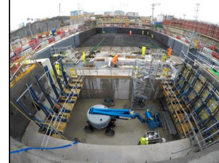
Conventional Island Unit 1 – Main Feedwater Pit
