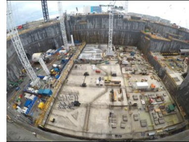
Heat Sink Unit 1 – Pumphouse
